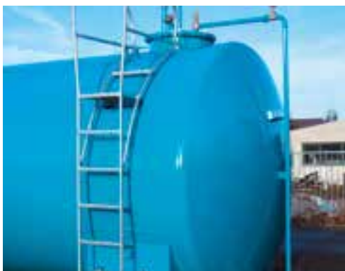
Diesel tank with platform and suction line
